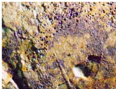
Metal surface after cleaning off rusts showing wide variation in pitted surface topography.
