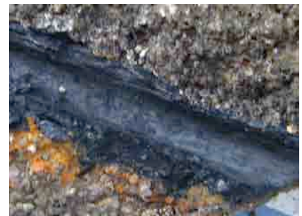
Anaerobic marine corrosion of reinforcing bar recovered from 65-year-old concrete structure.
